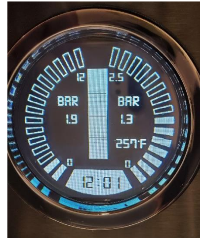
Steam Boiler Water Level Filled
